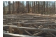
Truss joist systems require approved truss plan on site.
